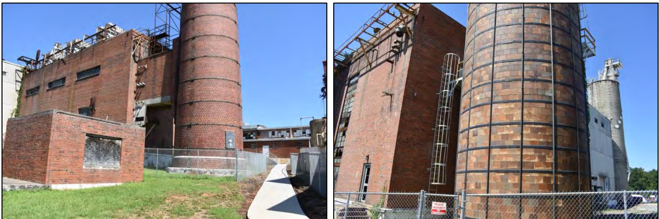
Figure 135: At left, south and east elevations of powerhouse, including base of smokehouse; at right, east and north elevations with tile and concrete coal silos
